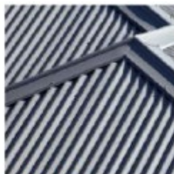
2 Metal Roof COLORBOND CUSTOM ORB PROFILE COLOUR: SHALE GREY SKYLIGHT FRAME TO MATCH
